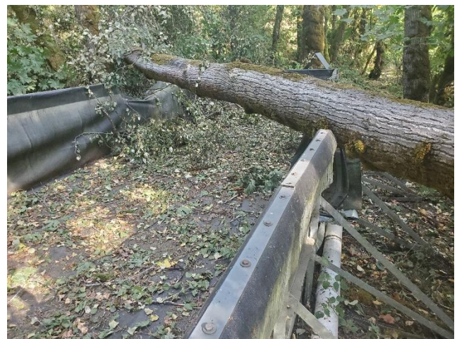
Tree damage at the Foster Creek acclimation facility
